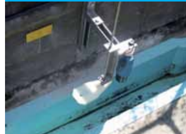
3107 Open channel flow
