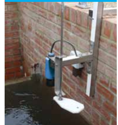
3108 High accuracy flow over weir
