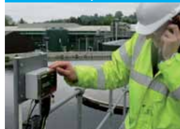
433S Sludge interface level
