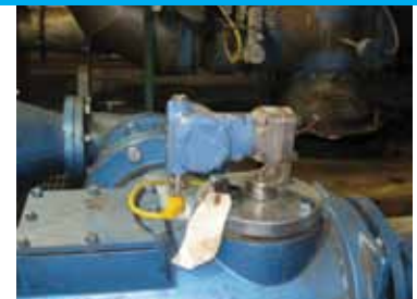
2051 Sludge pump pressure
