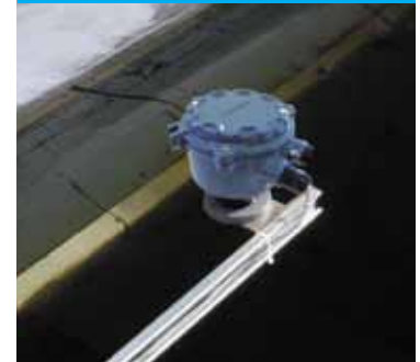
3100 Contact tank level
