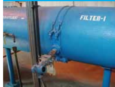
485 Annubar air flow to aeration
